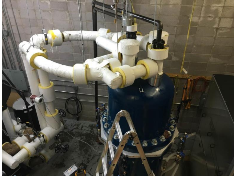
Figure 14. The 25 kW ThermoHeart Engine connected to the hot and cold plumbing.
