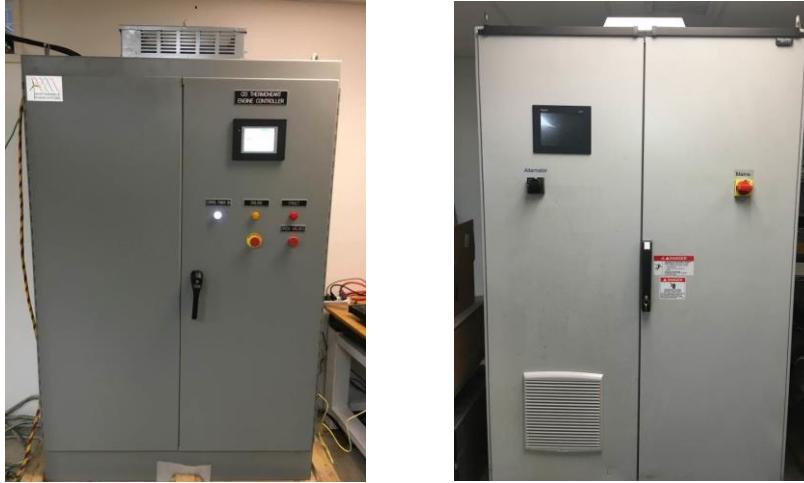
Figure 15. Engine controller/inverter system provided by Sustainable Power Systems in operation (left) and the Schneider Electric system in operation (right).
